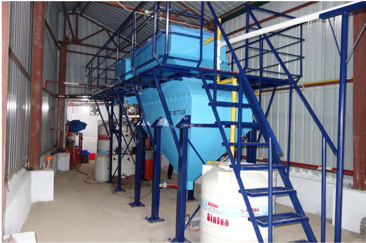
Arsenic removal Tube Settler.
