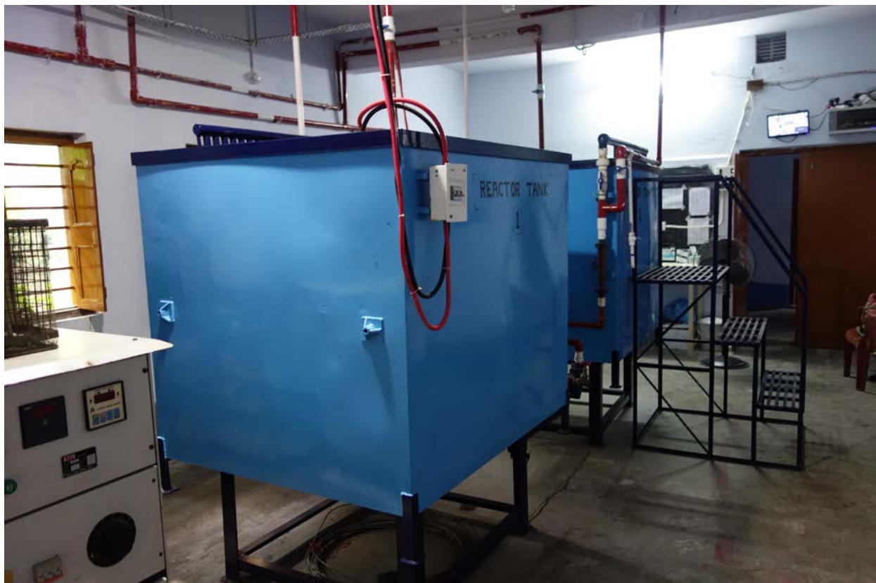
Arsenic removal Reactor Tank.
